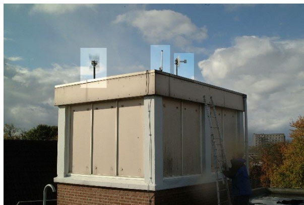
Figure 3: Antennas as mounted on a building (2 directional antennas and one omnidirectional antenna).
